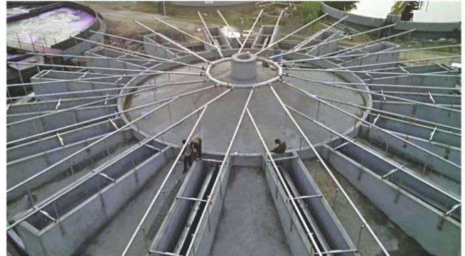
Process Utility Piping Systems
